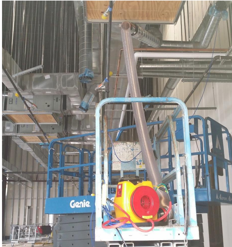
Figure 11 Model 400 Blower set up to test ducts prior to installation of the Flow Plug that is needed to measure flow.
