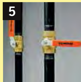
5 Render all stored and residual energy safe
