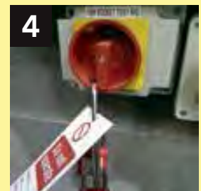
4 Application of Lockout/tagout devices
